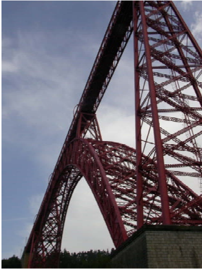
Figure 2. A close-up view of Garabit Viaduct shows level-3 shape-hierarchy. At level 1, we have the arch shape and we see criss-crossing beams at next two levels with smaller sizes just like in the Eiffel Tower.
